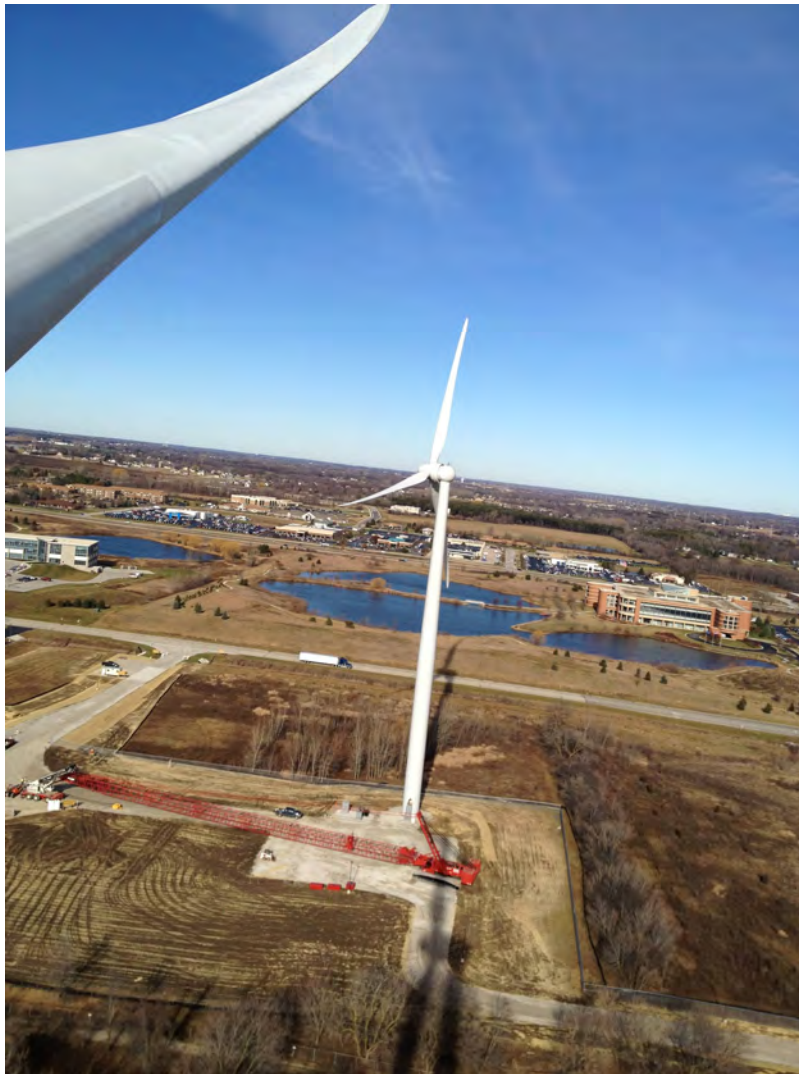
View of North Turbine from South turbine, main crane boom has been lowered
