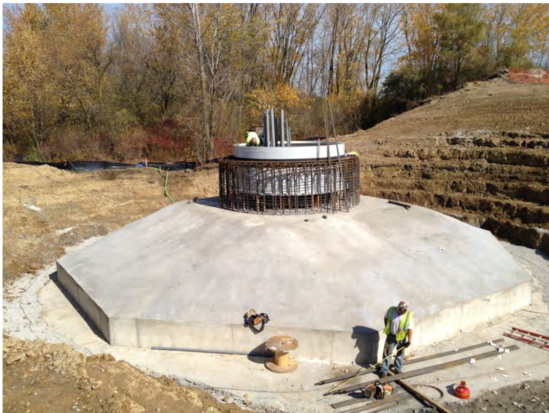
Foundation South turbine- included geopiers and larger mass to address poor soils
